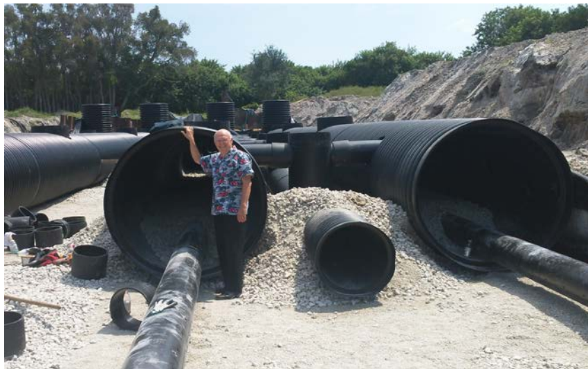
Figure 39. Up-Flow Filter in a Pipe
