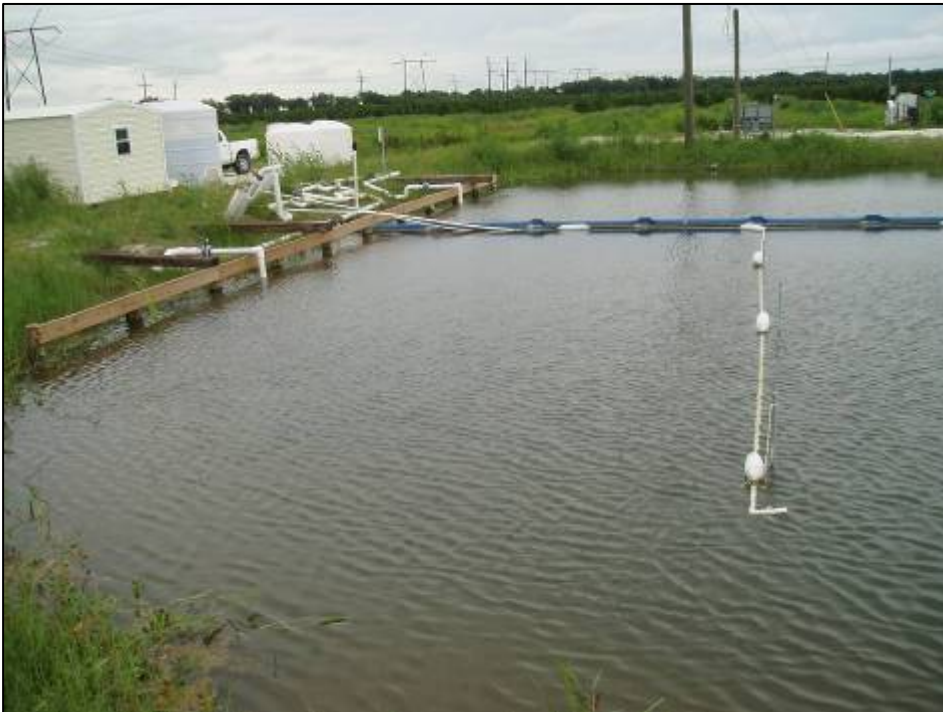
Figure 8. Floc recirculation infrastructure on the southern (B) HWTT flow path.
